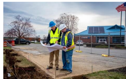
A Chase Bank installing an EV Charging station after completing a solar roof system
